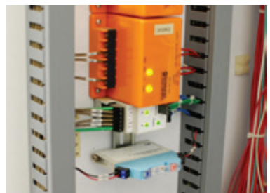
Zerust ActivPak protects expensive controllers in a panel inside of a waste water treatment plant.
