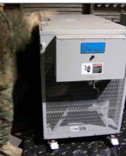
A portable load bank being positioned on a Zerust® ICT®520-XF Film Cover.
