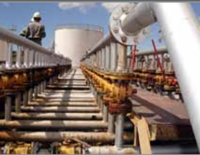
Rusted flanges without protection.
